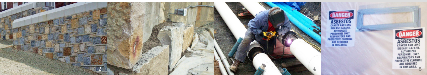
Photo 2: East retaining wall now complete. Photo 3: Recessed lights and stone veneer installed at the amphitheater. Photo 4: Contractor makes welds on hot water lines. Photo 5: Procedures in place during abatement activity.
