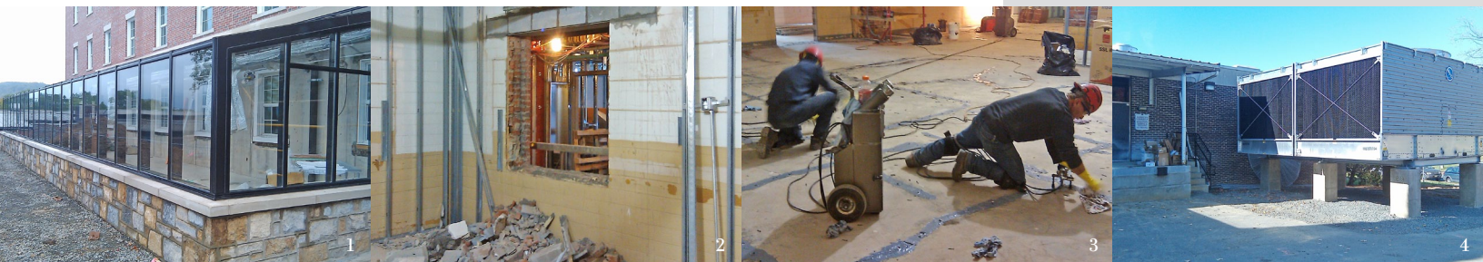
Photo 1: New greenhouse. Photo 2: Selective Phase 2 demolition and rough-ins. Photo 3: Contractor remediates structural cracks throughout existing floor slabs in Phase 2. Photo 4: Central Plant cooling towers
