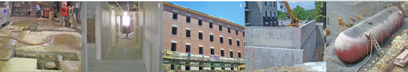
Photo 2: Floor drain installation in the Campus Center mechanical room. Photo 3: Drywall work continues in the Science Center. Photo 4: Brick installation on the west side of the Science Center. Photo 5: East retaining wall. Photo 6: Water-retention tank installed.
