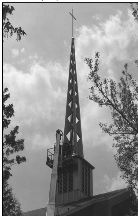
MPK Memorial Chapel's steeple is back in place after the structure broke early this year. Photo by Andrew Holets
