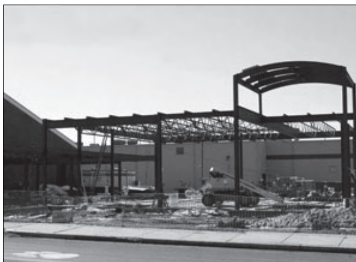
Photo provided by Albright website Schumo Center construction still under way and on schedule.
